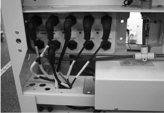
Figure C-12: Cables under cross beam and attached to analog module
