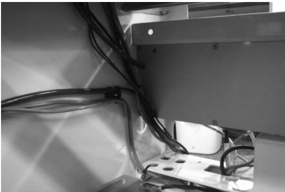
Figure C-9: Cables running down inside HCGG towards the modules
