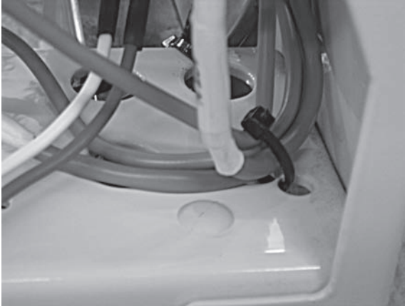
Figure C-10: Cables secured to frame with tie
